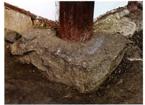
동금강암 앞면 동쪽 귀기둥 주춧돌 東金剛庵 前面 東側 隅柱 礎石 plinth for front eastern corner column, Tonggümgangam
