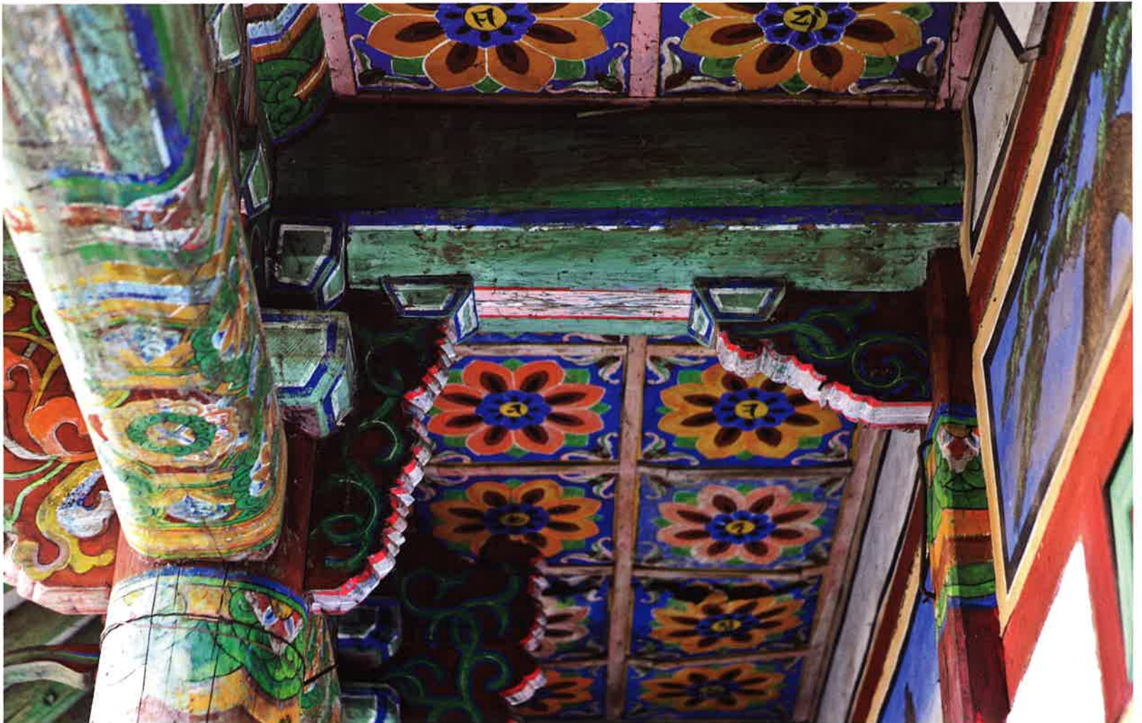
동금강암 뒷간 주상포 / 東金剛庵 退間 柱上包 brackets above columns of space with extra poles outside the inner fence, Tonggūmgangam
