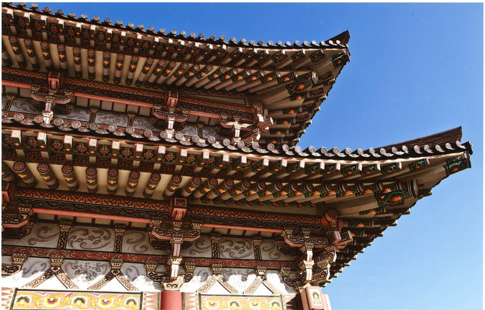
보광전 1, 2층 처마와 공포 / 普光殿 1, 2層 軒·栱包 / 1st, 2nd floor eaves and brackets, Pogwangjŏn hall
