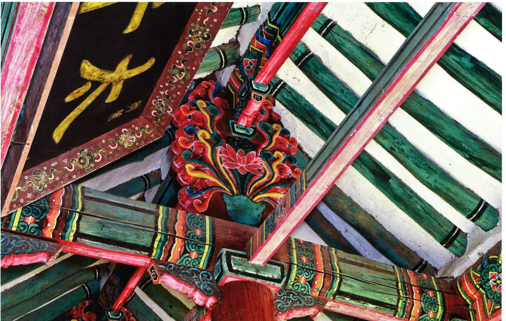
태평루 앞면 화반대공 / 太平樓 前面 花盤臺工 / short pillar to hold purlins of Hwaban, Taep'yongnu
